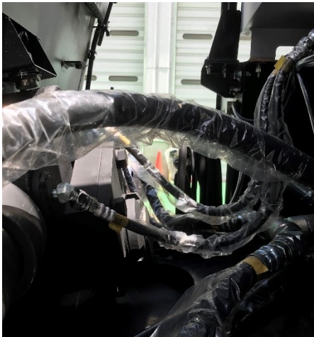
Pump unit valve
